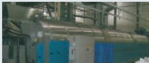
Simultaneous Chemical Delivery Service to Tunnel "CBW" Washer Modules
